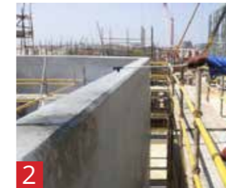
2 Moisture Control The principle of controlling moisture with acceptable levels using coatings and membranes.
