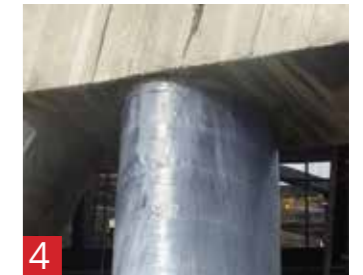
4 Structural Strengthening Replacing lost strength or increasing strength by adding steel, additional reinforced concrete or Fibre Reinforced materials.
