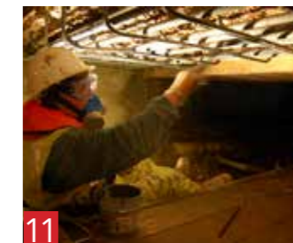
11 Control of Anodic Areas Corrosion of the reinforcement is controlled by a complete film formation, using coatings or corrosion inhibitors.
