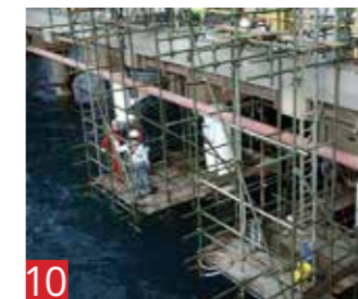
10 Cathodic Protection Cathodic protection manages the output of current through the steel to channel currents to specific anodic sites. This may be done using external currents or sacrificial anodes.
