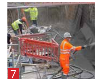
7 Preserving Restoring Passivity Using mortars or concrete to replace contaminated concrete. Also techniques for re-alkalisation and chloride extraction.
