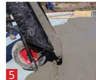
5 Increasing Physical Resistance Replacing lost concrete or providing additional cover and protection.
