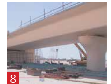
8 Increasing Resistivity Using coatings and protective systems to reduce the level of moisture in the concrete thereby increasing the electrical resistivity of the concrete and reducing the potential for corrosion.
