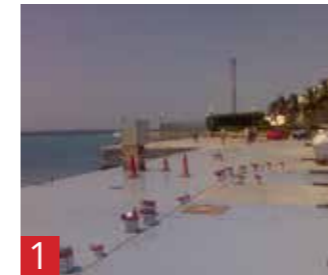
1 Protection against Ingress The basic principle is to keep the concrete dry by reducing its permeability by closing up pores and cracks.
